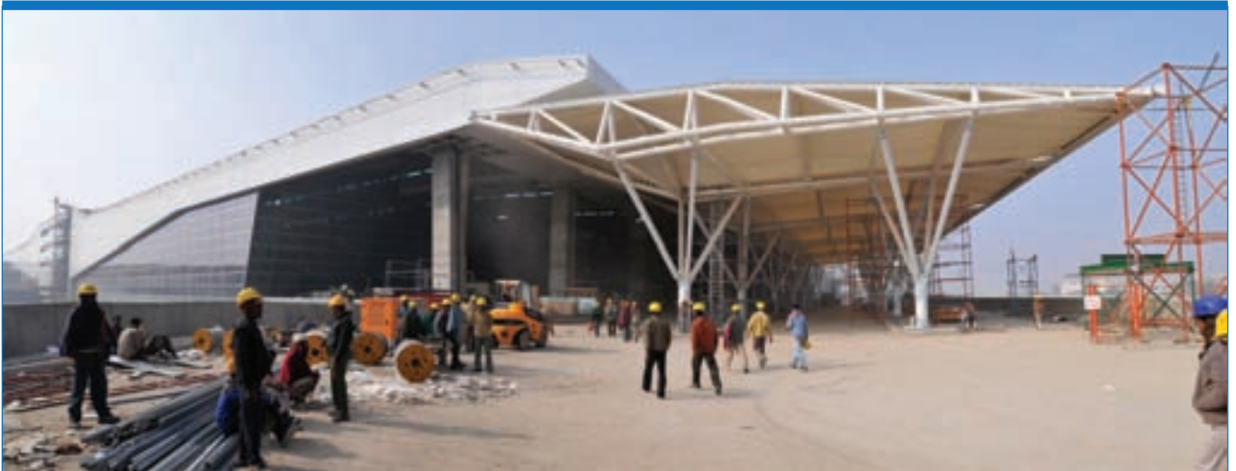
Construction of Indira Gandhi International Airport's Terminal 3 is under budget and ahead of schedule.
